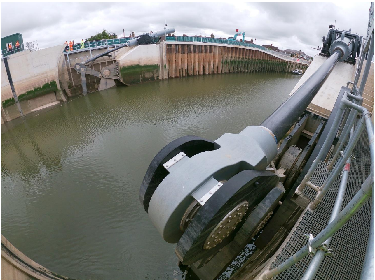
Hydraulic cylinders in open gate position
